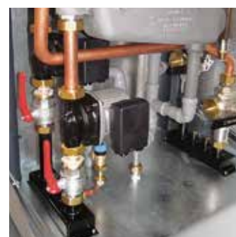
Pumps and gate valves
